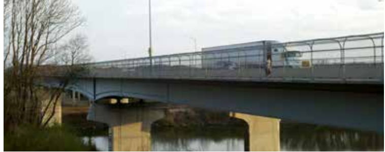
The Singing River Bridge between Muscle Shoals and Florence is a critical connector within the regional bicycle and pedestrian network.
